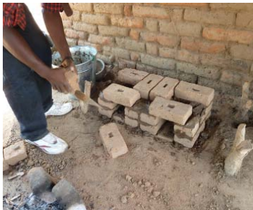
Assemble the bricks like this and use the mud mixture as a mortar between the bricks and between each layer
